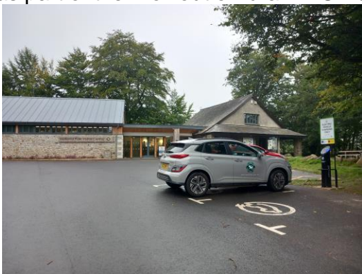
Charging point at Postbridge VC
